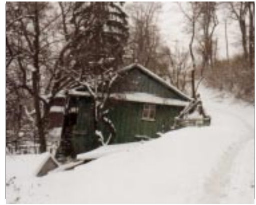
With its foundation sliding downhill, this house is now leaning about 8 to 9 degrees from the vertical.
