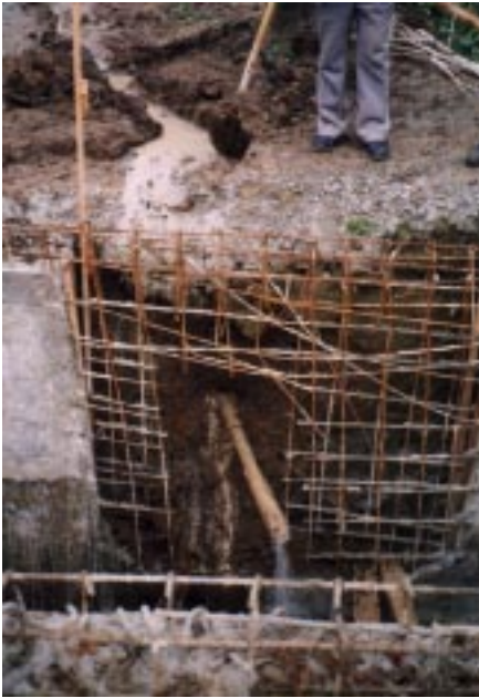
Drill exits at bottom of hill dead center in exit pit cut in retaining wall.
