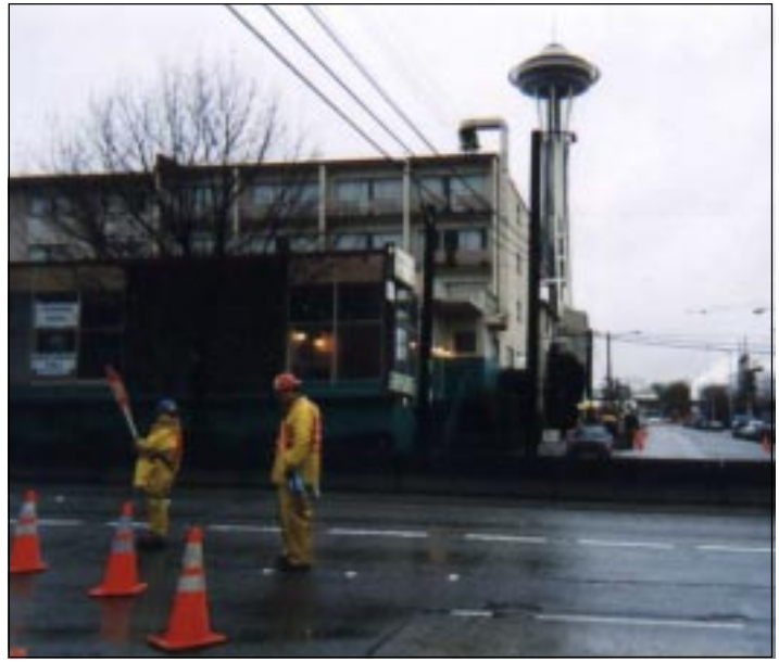
Crew monitoring traffic on Aurora Avenue in Seattle. Note drill rig across highway near base of Space Needle.
