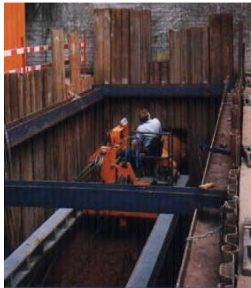
Thrust frame at end of stock; note cutting spoils under frame and rails.
