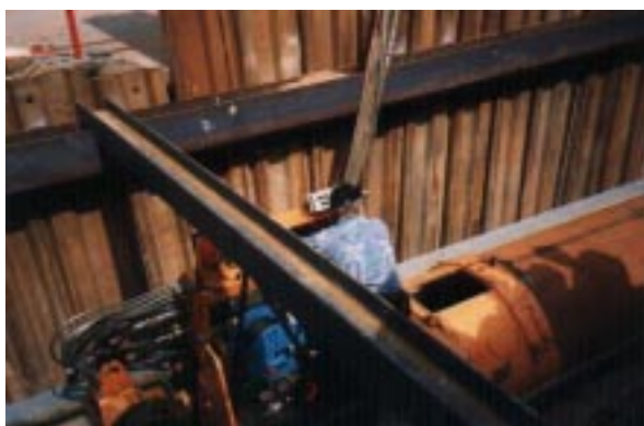
Operator on thrust frame viewing Remote Display and cable at exit of protective casing.
