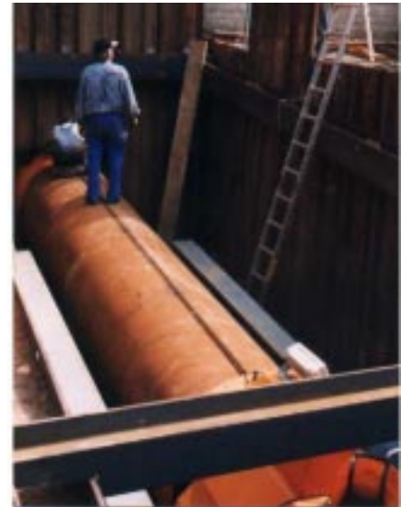
Casing with path for cable on top.
