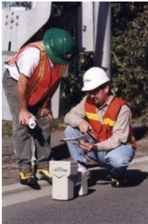
DCI's Soggi Finsson and Joe Zeck using the new DigiTrak Eclipse System.
